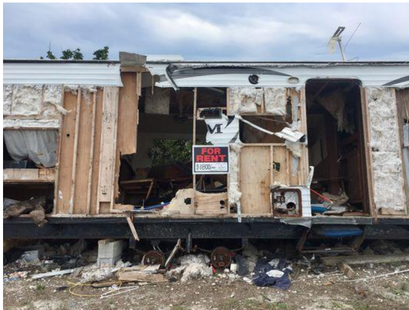
A "For Rent" sign hangs on the remnants of a trailer damaged by Hurricane Irma on Sugarloaf Key, Fla., on March 9, 2018. Affordable housing has reached crisis levels throughout the Keys following Irma as working-class residents are struggling to find places to live. (Photo: Alan Gomez, USA TODAY)
